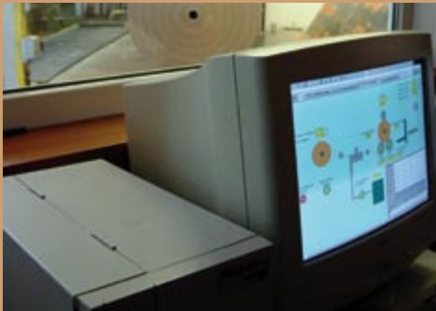
Final Control Process Station
