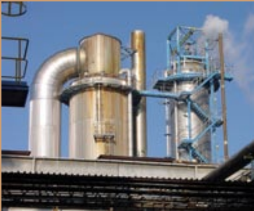
Pulp processor system at Mondi Packaging
