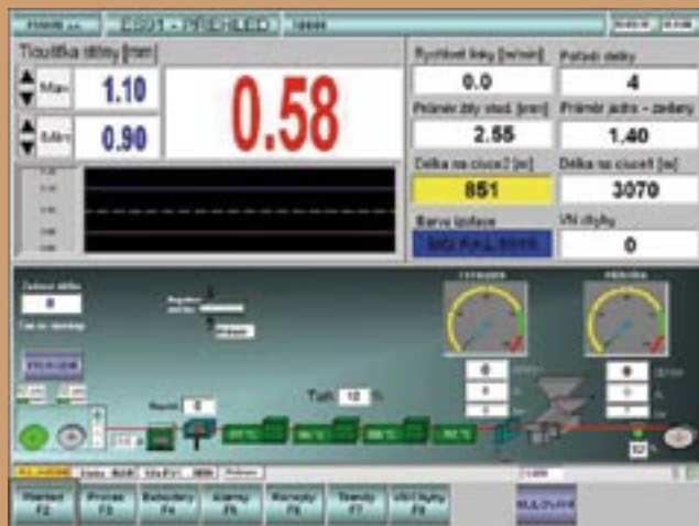
Main Control Screen at PRAKAB a.s.
