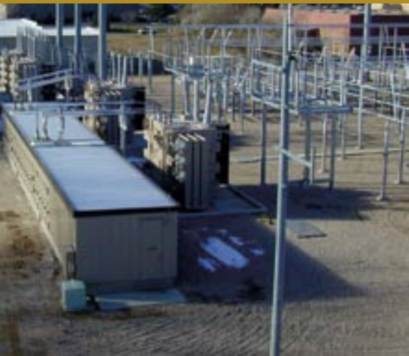
A Fort Collins Utilities Monitored Substation
