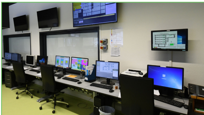
CALA Control Center Photo Credit: Mesalogic
