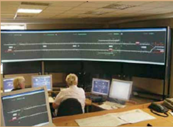
Dispatching Desk at Kazan Metro Operations
