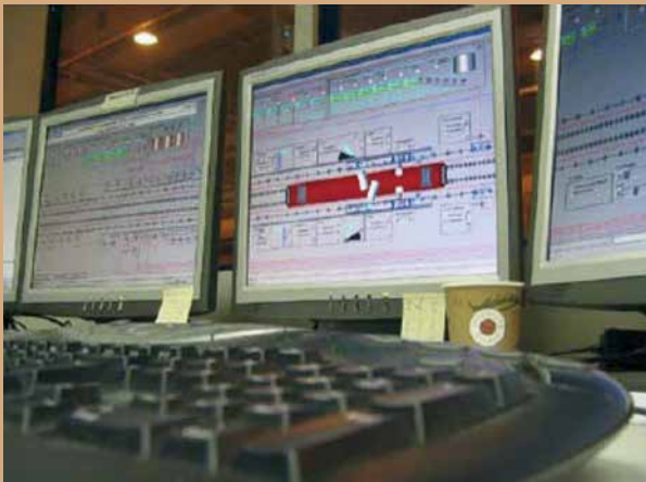
Train Wash Operator Control Area
