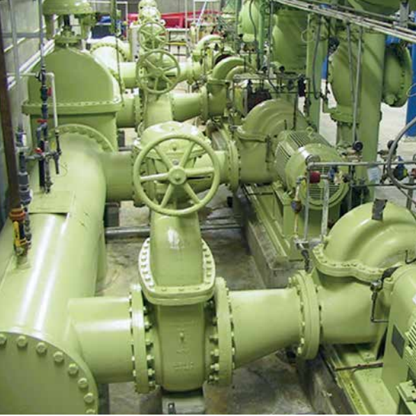
Water Pumps at Keokuk Municipal Water Works
