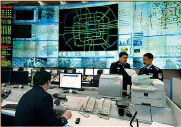
Monitor/Control Room within the Beijing Traffic Control Center
