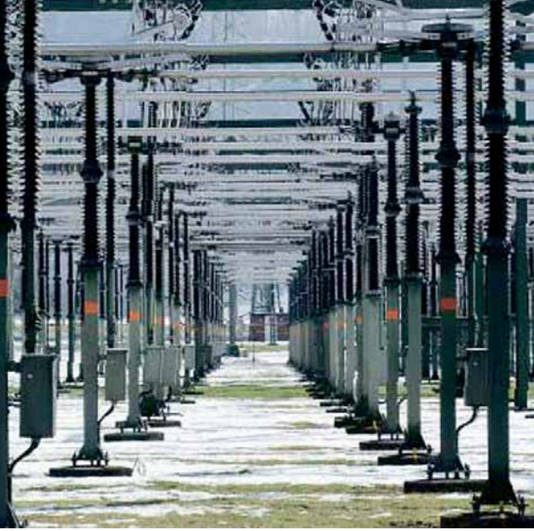
Power Transmission Lines Switzerland
