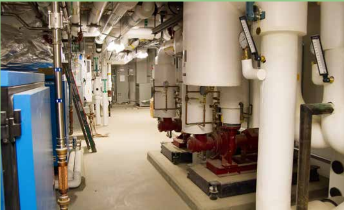
A Campus Building Mechanical System Monitored by GENESIS64™
