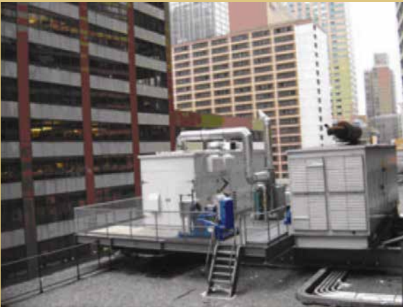
A DFC300 Installation in Downtown Manhattan
