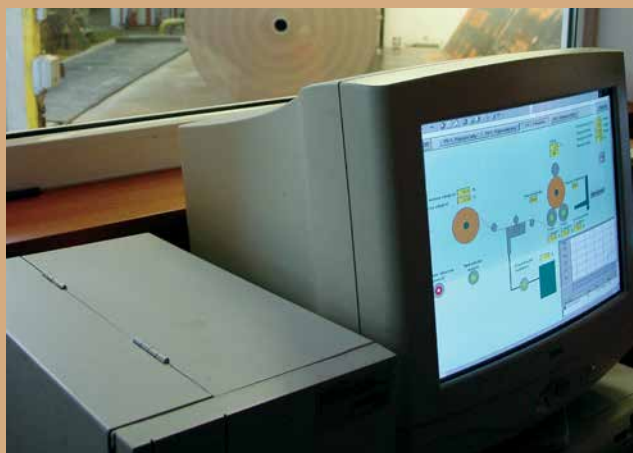
Final Control Process Station
