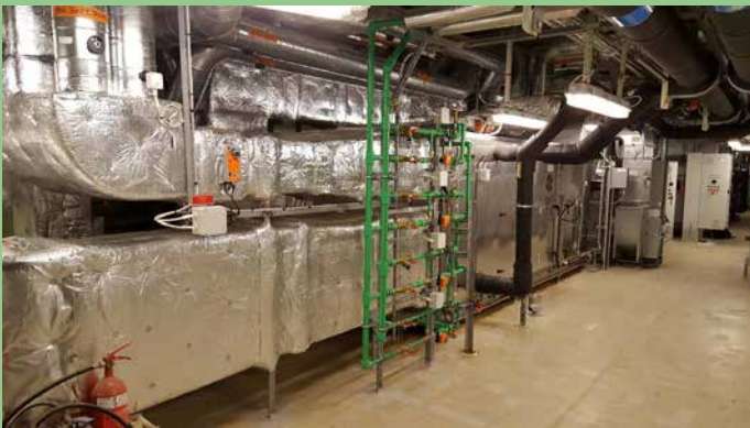
An MSC Meraviglia HVAC System
