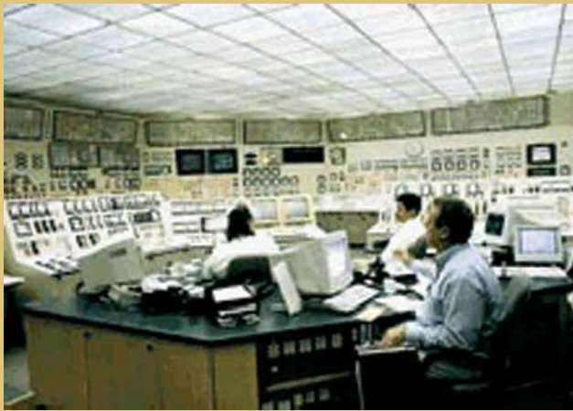
Plant Control Room at Ameren Callaway Facility
