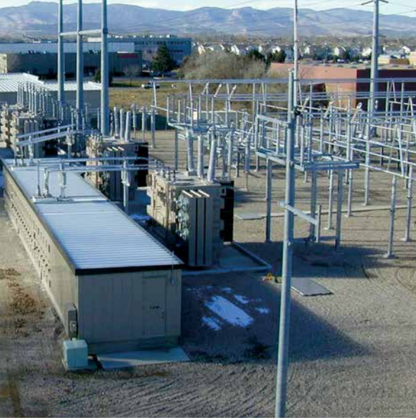
Fort Collins Utilities Monitored Substation
