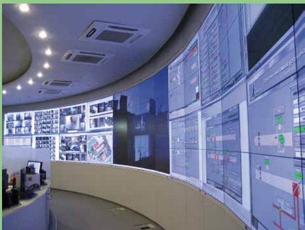
HMI/SCADA In Action at the Federation Tower (West)
