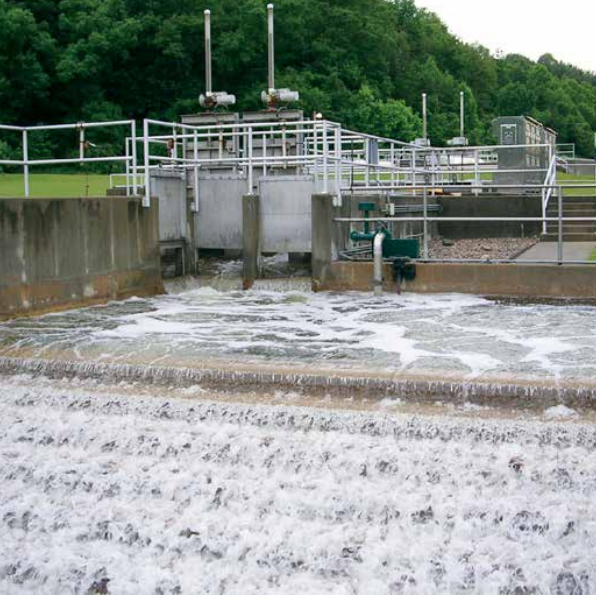
Water Treatment Plant in Operation
