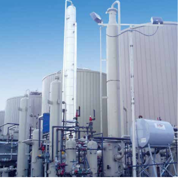
Microgy's Digester Equipment
