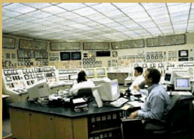
Plant Control Room at Ameren Callaway Facility
