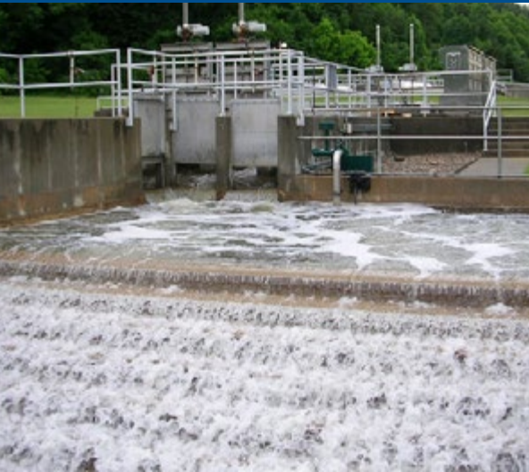
Water Treatment Plant in Operation
