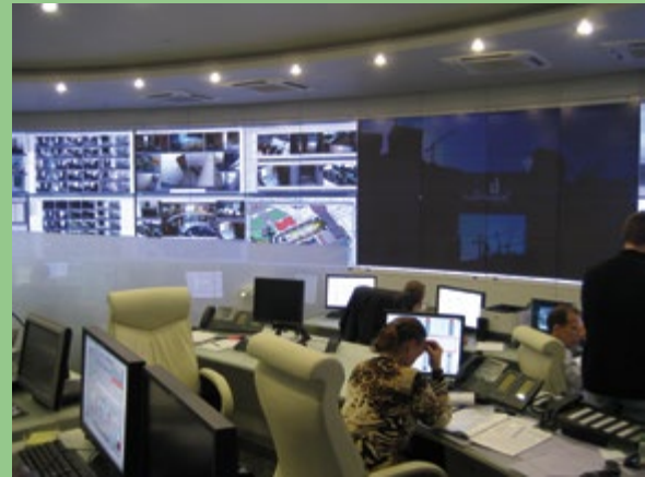
The Building Control Center Inside the Federation Tower (West)
