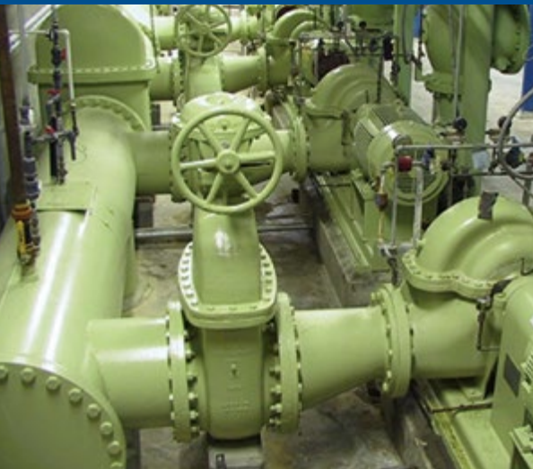
Water Pumps at Keokuk Municipal Water Works
