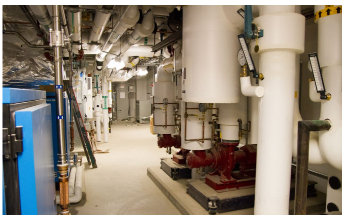
A Campus Building Mechanical System Monitored by GENESIS64™
